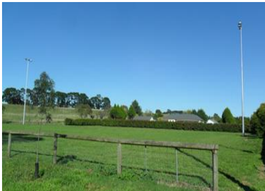
Taralga Sports Oval Flood Lighting Project - supply and erect a pole mounted flood lighting system
